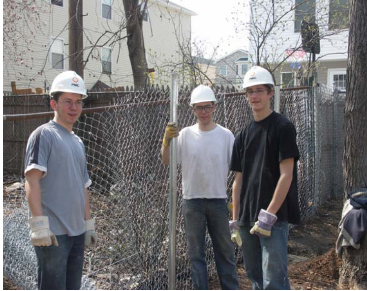
Three of the boys work to place fence posts in the ground before the fencing materials can be hung. The students worked on a variety of different projects during their two week visit to HFHN.
