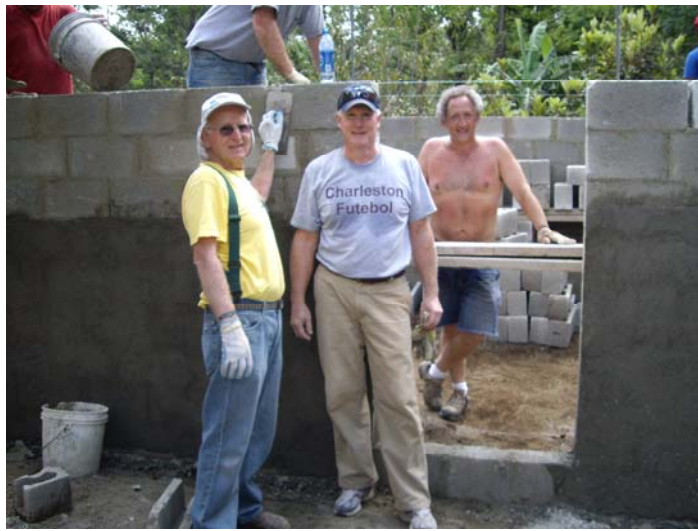
Near the end of day #3 the walls are starting to take shape and you see Jim Tierney and Jim Fehon taking a photo break in front of the soon to be home.
