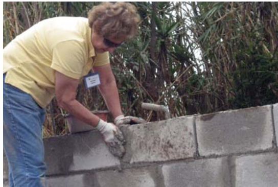
Jeanne Scott works mortar in between the cinder block to make sure the new house is tight and solid.
