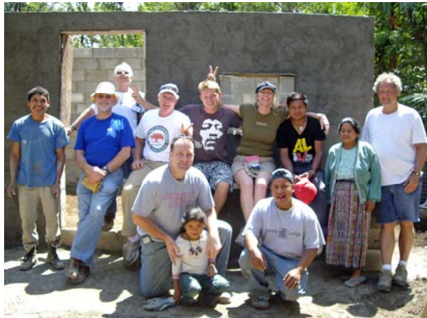
It took a crew of seven volunteers, the new owners and two staff builders from From Houses to Homes but as you see the building has topped off and now ready for a roof.
