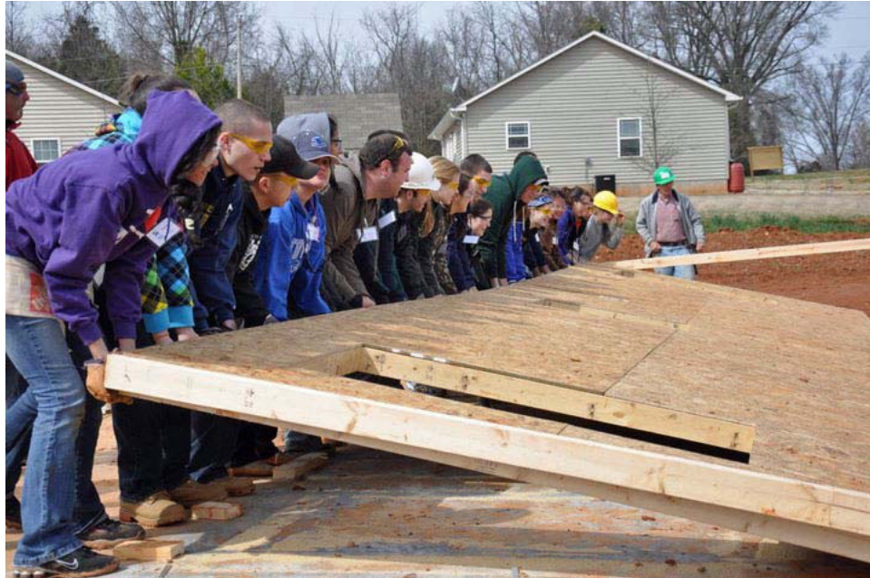
Everybody lift now! A wall goes up on a home in Davidson, NC where students From Seton Hall University Habitat for Humanity Chapter spent their Spring Break helping build a home for a hard working low income family.
