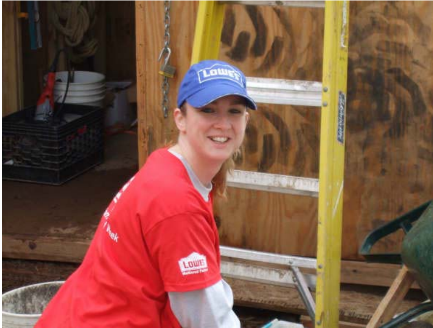
Kathy McFadden prepares to climb the ladder and work on siding the Habitat Women Build House.
