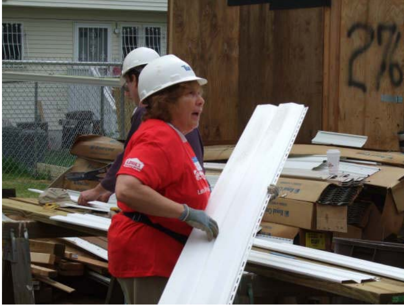
With a piece of siding cut and ready to go Sheila Wolfensohn of Florham Park heads to the installers to out it in place.
