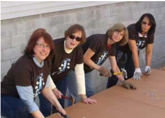
Putting the outside sheetrock on one of the first walls to rise for the Women Build III house are (left to right) Carol Paster (Co-Chairperson of Women Build), Suzanne Sullivan, Gail Laughlin and Rosie Jaworski.
