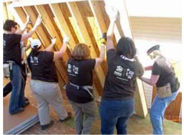
Up goes the wall section for the first floor of Women Build III House in Newark. Guiding it into place are (Left to right) Lisa Kelly, Virginia Petrucci, Sheila Wolfensohn, Rosie Jaworski and Jane James.
