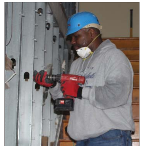
Corporate Challenge teams work on a Critical Repair project in Jersey City. Top: TD Ameritrade. Bottom: Anheuser-Busch.
